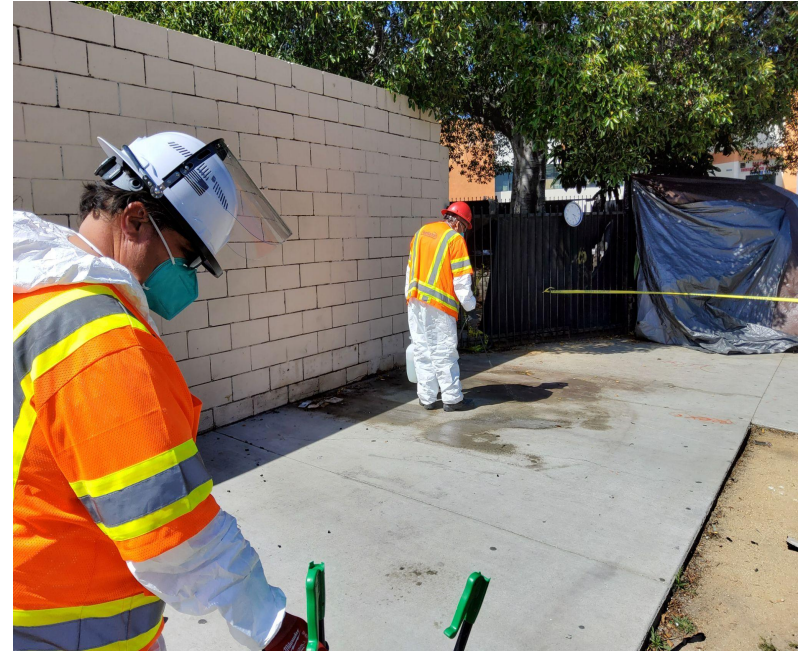
PHOTOS FROM CITY OF LOS ANGELES BUREAU OF SANITATION AND ENVIRONMENT
